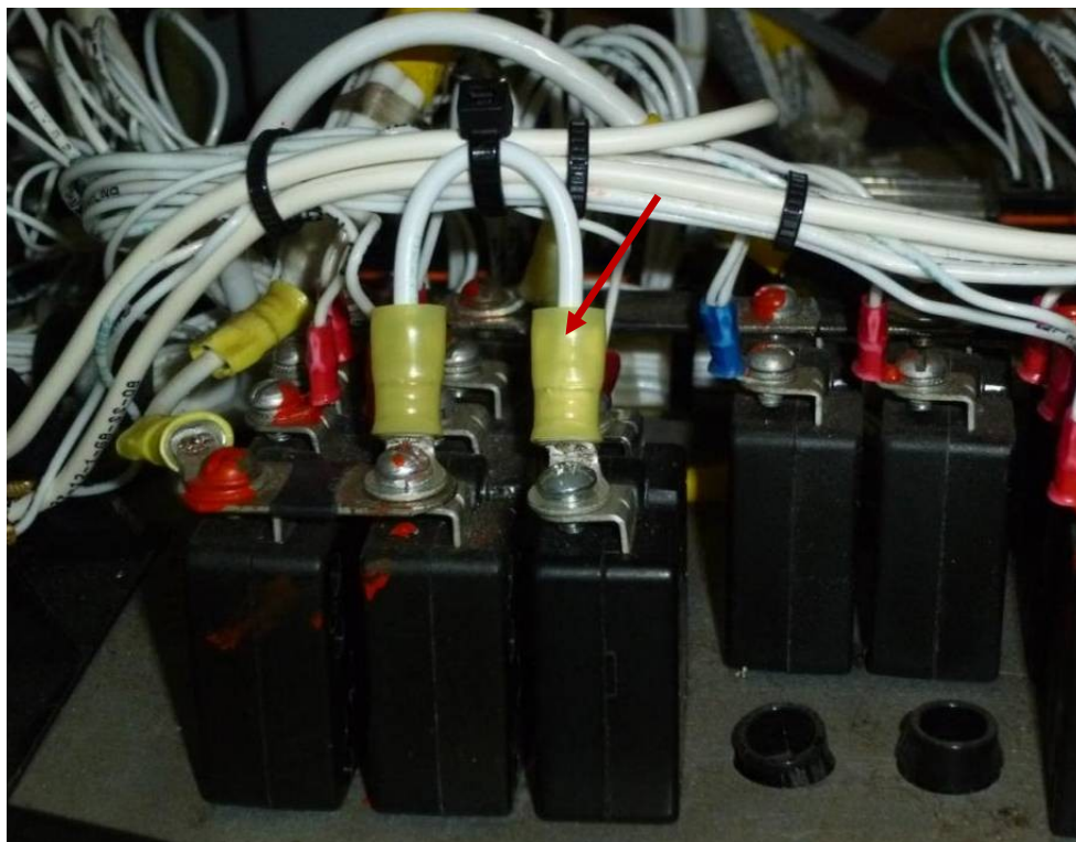
Figure 3 Connection of Circuit Breaker to Main Bus Bar
