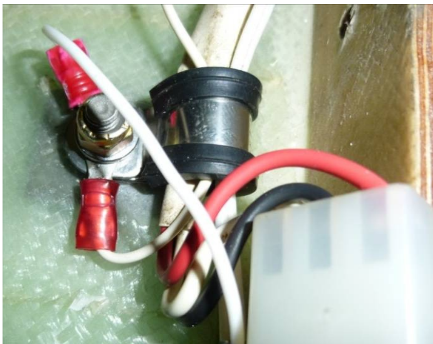
Figure 9 Connection of cables and attachment of loose cables to bolt with clamp
